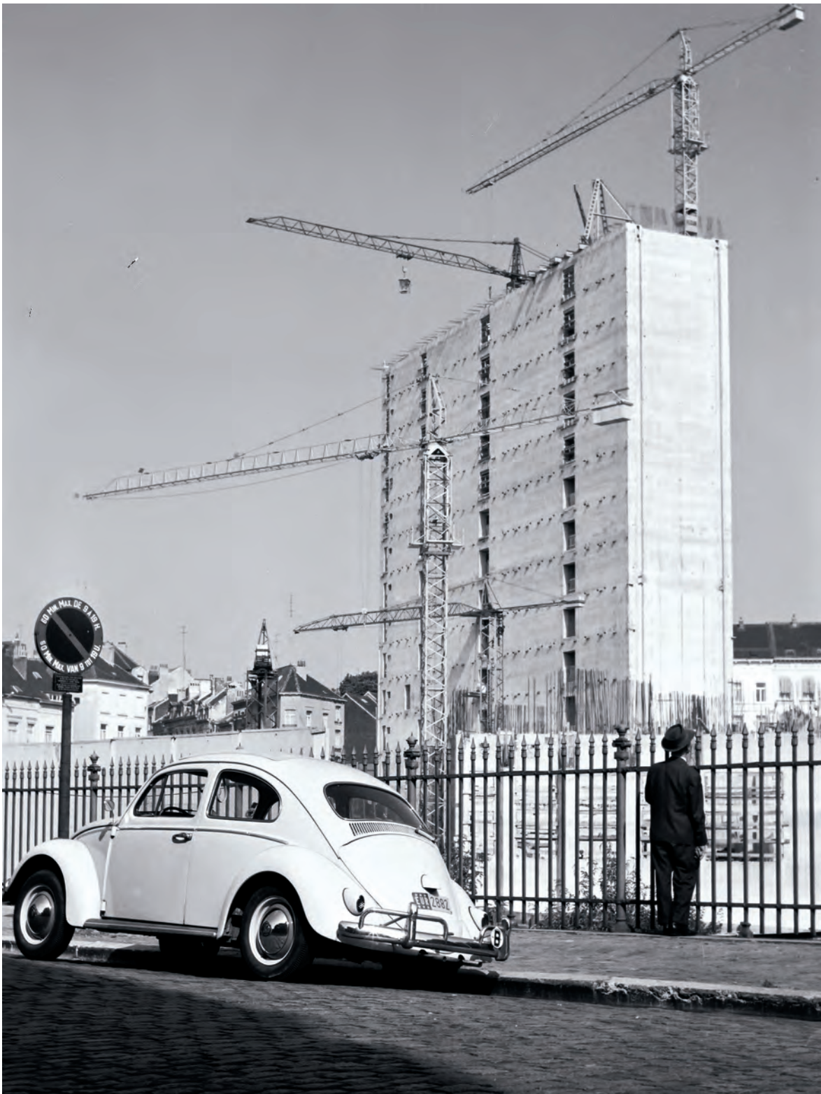
Brussels, 30 September 1964, Berlaymont under construction. It is built wing by wing. Originally scheduled for 1964, the first wing is completed only in 1967. The Directorate-General for Agriculture settles in there.
